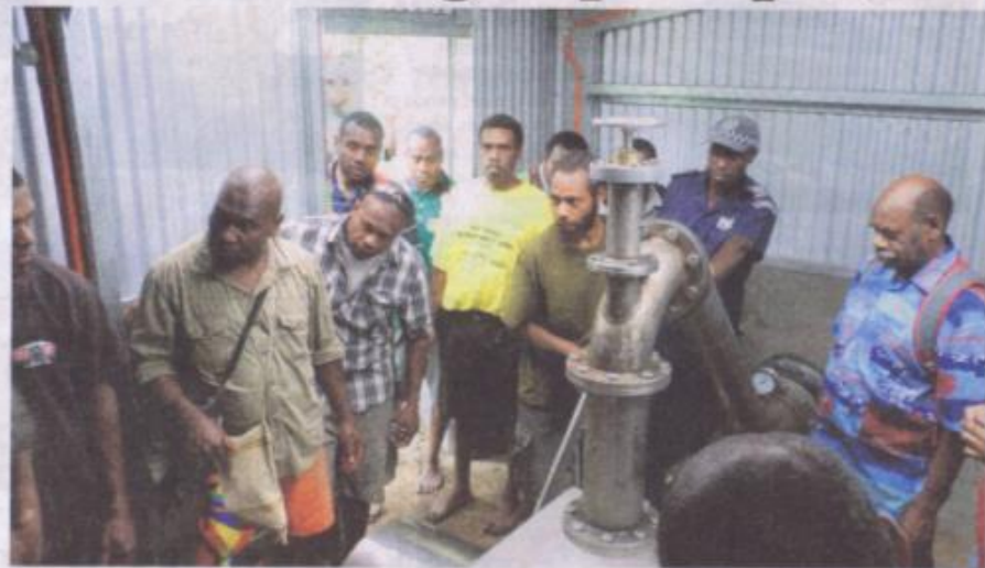
LEAP FORWARD: Vanuatu officials and residents inspect the Dorrigo-built turbine and control system installed in Talise Village at an official start-up last week.
