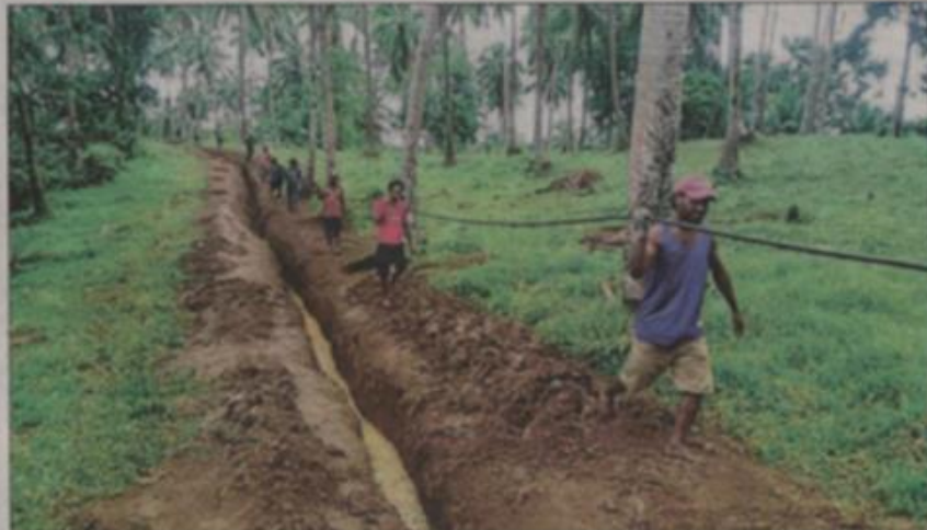
Local helpers carrying HV cable from the village of Tam to step up
